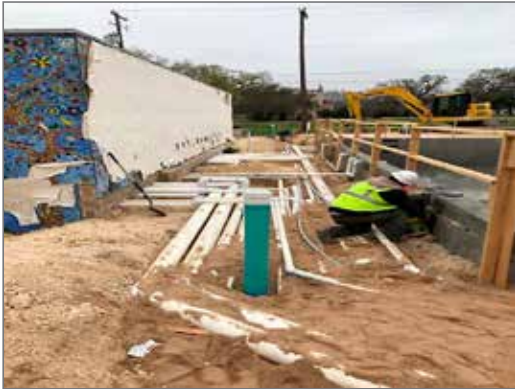
Plumbing from Pools to Mechanical Room
